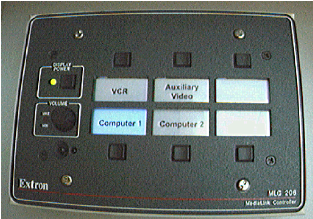
Extron Control Panel
